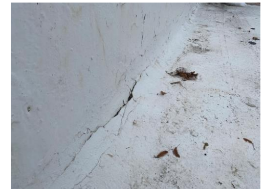
Pool surface cracking
