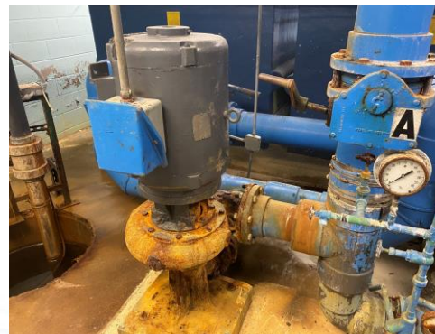
Mechanical equipment corrosion
