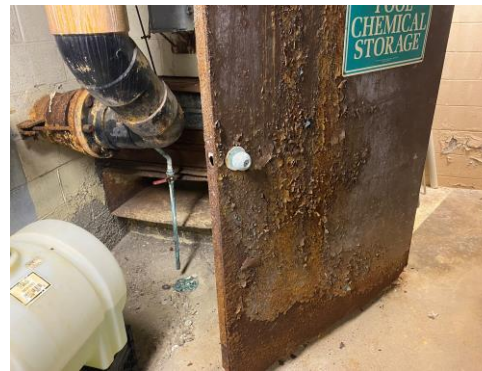
Mechanical room door corrosion
