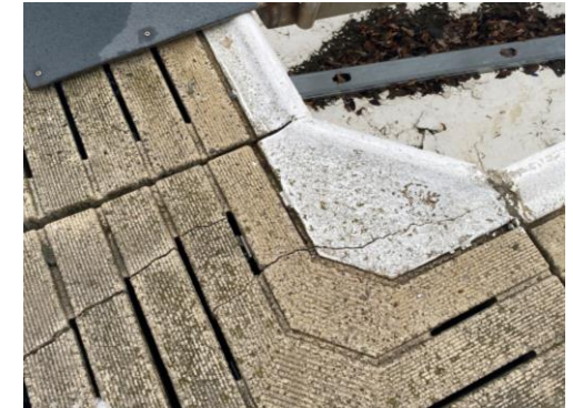
Cracking in gutter system
